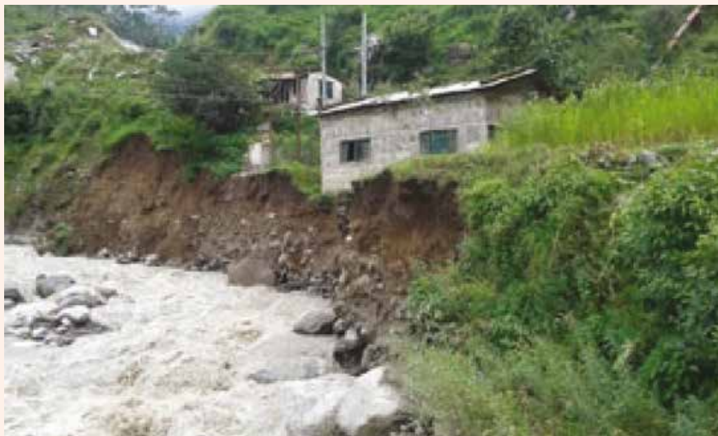
Figure 4 Power house of the Triveni Micro Hydropower Project at risk by the Bahuli Rivulet, in Martadi of Bajura (Source: Prakash Singh) http://www.the-himalayantimes.com/fullNews.php?headline=Bajura+headquarters+in+dark+for+five+days&NewsID=424456#sthash.77OQPrqW.dpuf
