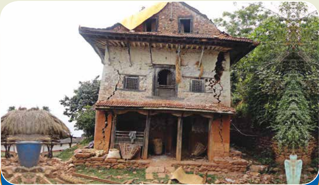
A Rural House Damaged by Gorkha Earthquake
